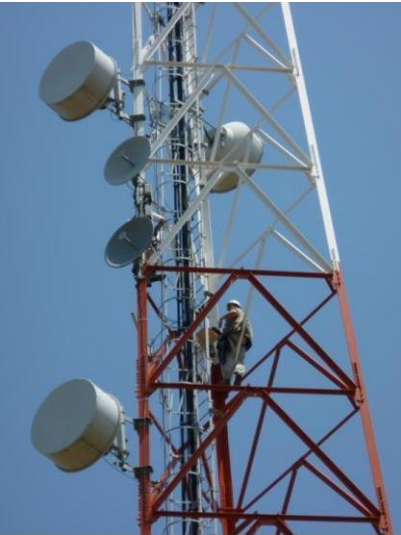
WiFi connection installed in Mangochi, Malawi
