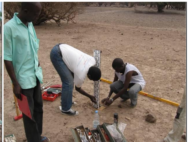
Photo 2 Limnometric scale installation Niaka pond
