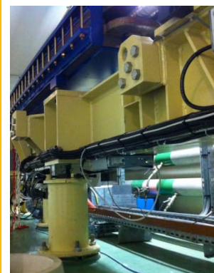
Libera Spark instrument installed inside the booster tunnel
