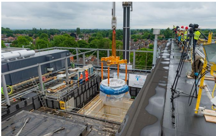
State of the art cancer-treating cyclotron arrives at The Christie in Manchester, UK. (Image credit: The Christie)
