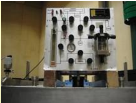
Gas control station
